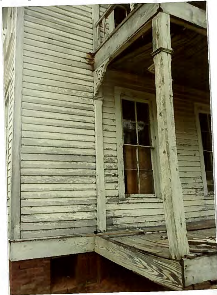
Deteriorating Condition of the Dr. Samuel Floyd Vaughan Home At the Time Samuel Floyd Vaughan III Gained Ownership in the Year 1983
