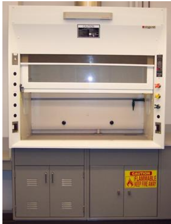
(Most hoods on campus are standard VAV hoods)
