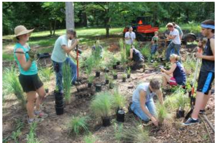
SFA Gardens student workers install plants in one of three new rain gar-
