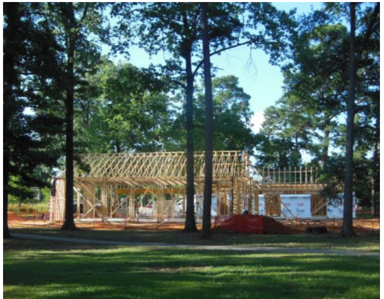
Construction of the new Conservation Education Center is well underway at the Pineywoods Native Plant Center
